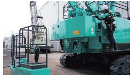
The counterweight can be assembled by operating the winch and raising and lowering the counterweight self-removal arm.
